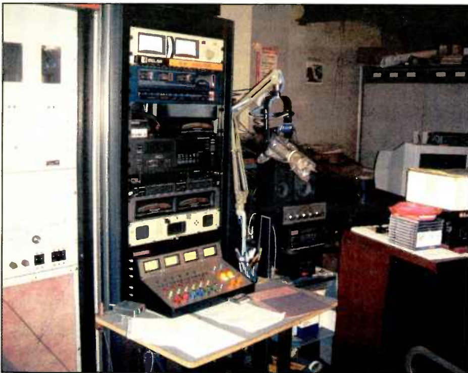
The transmitter room at the archival house.
