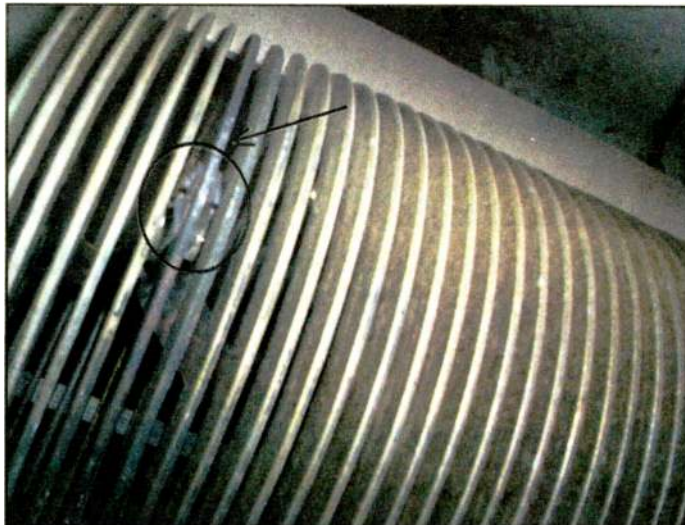
Fig. 2a: Close-up of defective coil tap.
