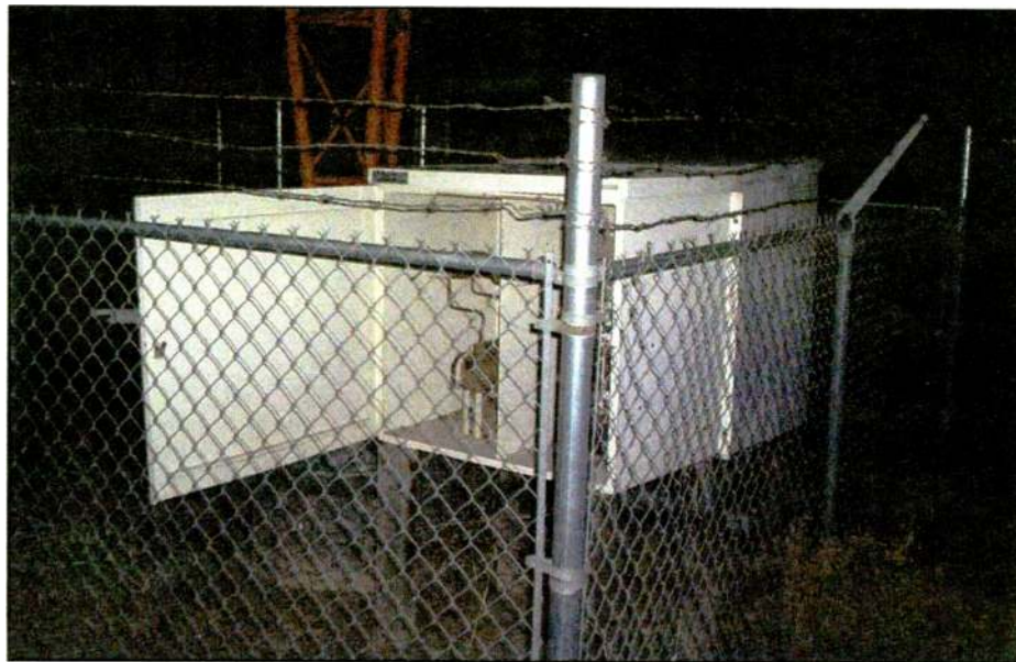
Fig. 1: This was how the ATU was found — with the ATU cabinet door wide open!
