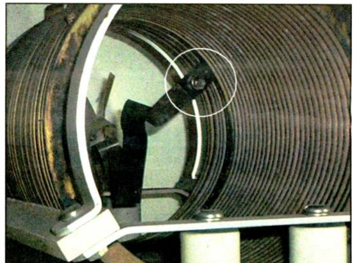
Fig. 2b: Defective coil tap as viewed inside the coil.
