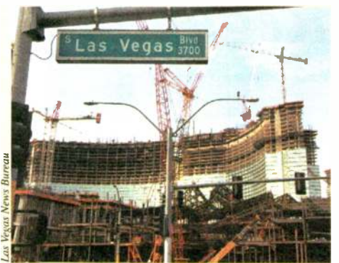
Construction continues on the massive MGM Mirage City Center, the largest construction project ever in Las Vegas, according to the LVCVA.
