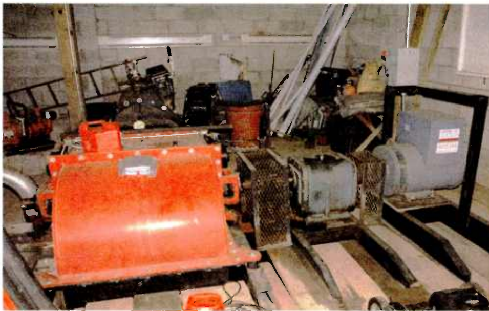
25 and 45 KW turbines in the powerhouse generate electricity to power the studio building. Excess power is sold to a utility.
