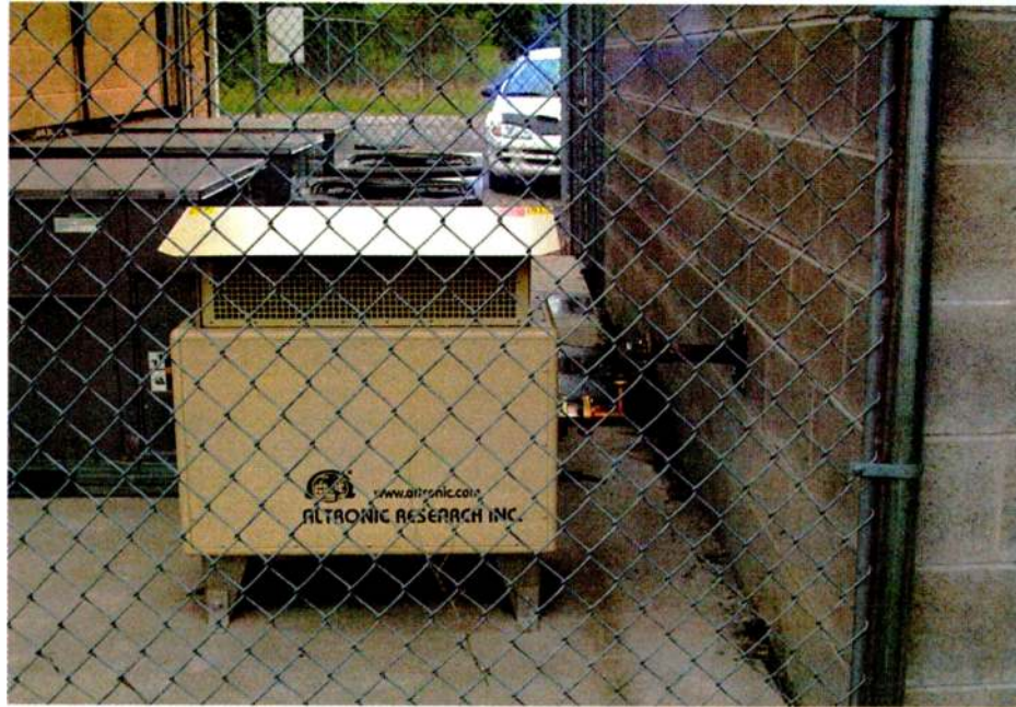
A reject load is required for high-level combined FM systems. Outdoor loads like this help with costs by keeping the heat outside.
