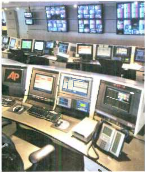
Master Control Room
