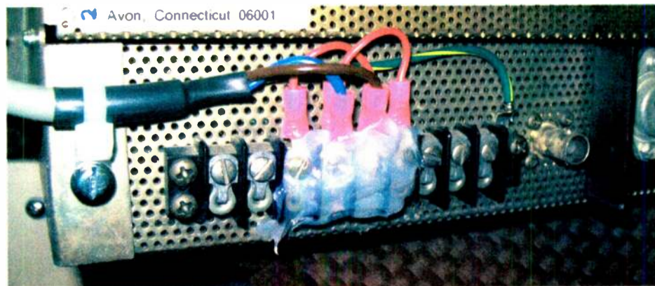
Fig. 4: Use clear silicon caulk to safeguard bare AC terminals.
