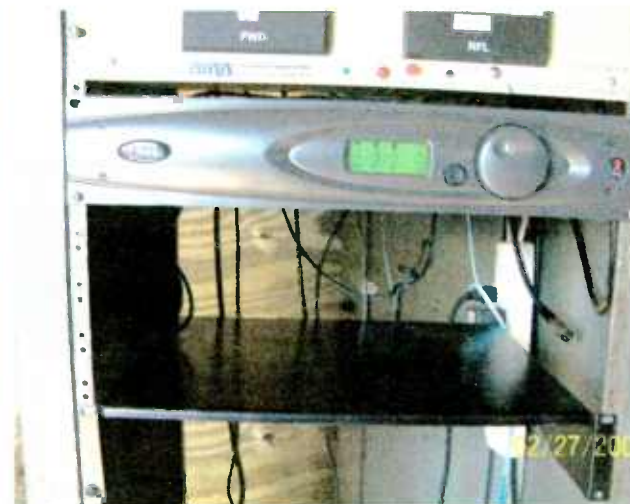
Fig. 3: Rack shelf in place after the exciter is removed.
