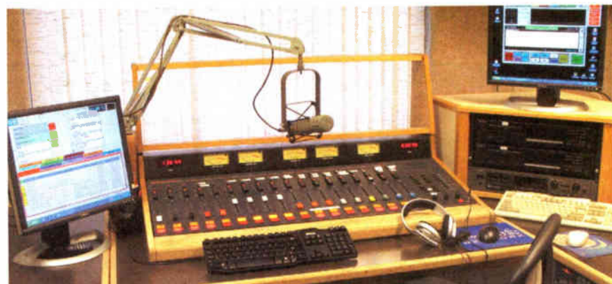
BE AudioVaults, networked via satellite, are serving Family Life Network, including this studio.
