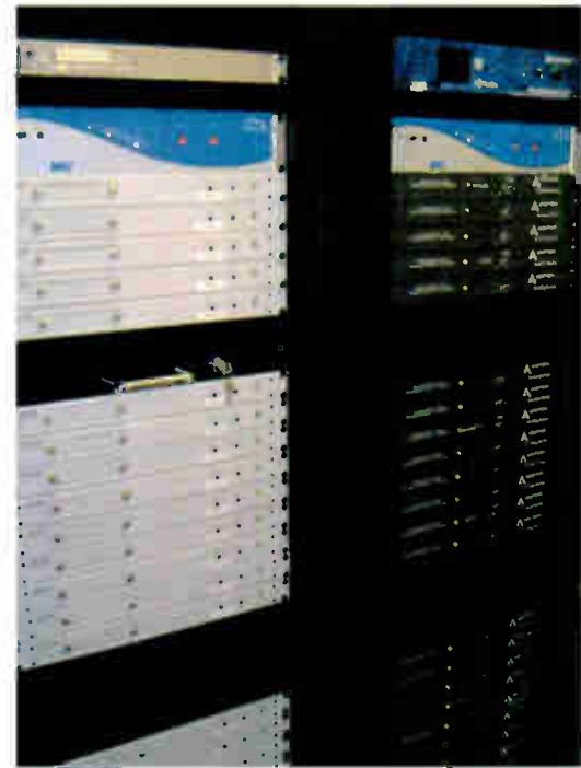
A portion of two racks of equipment monitoring silence and Arbitron PPM encoding on some of Greater Media's 22 audio streams in Philadelphia. From Larry Paulausky's presentation.
