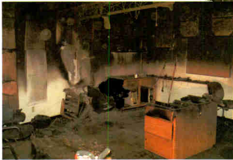
Studio 1 was a total loss from the latest fire.
