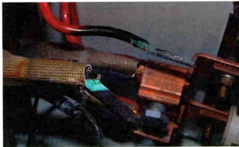
Fig. 2: Damaged wires after removing the lug.
