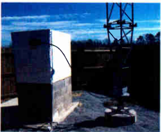
High-Power Antenna Tuning Units
