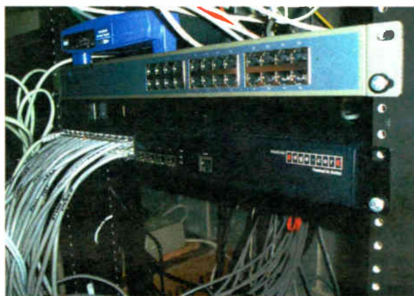
A 24-port ES4524D Edge-corE switch was installed by Small Tree Communications at WWIB(FM) in Wisconsin.
