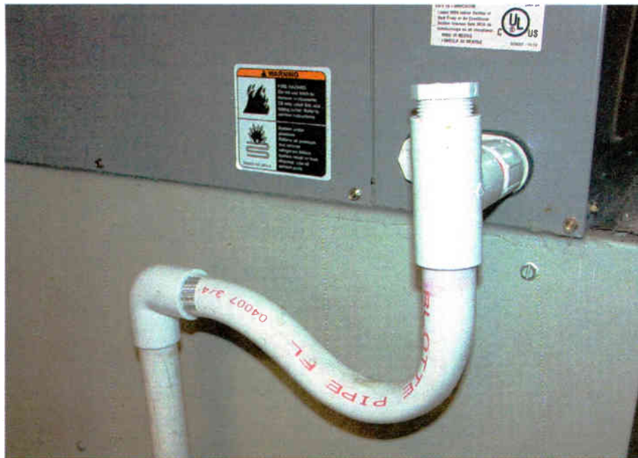
Fig. 1: Keep the condensate drain clear to avoid floods.
