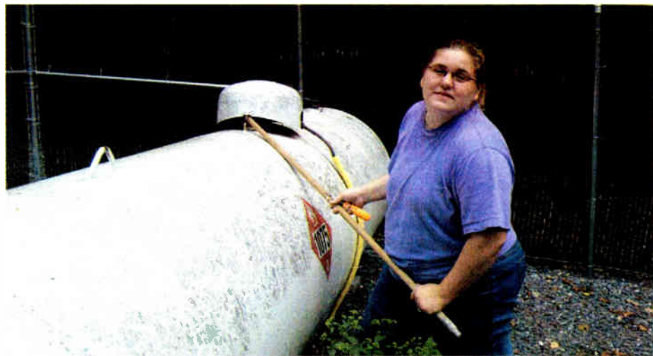
Getting ready to check the fuel level in the tank for the WGYS generator, part of weekly maintenance. "We have had some issues with wasps and hornets building nests in the cover on the propane tank so we are careful when lifting that lid," Timmons said. The easiest way to do this and not get stung: use a big stick!
