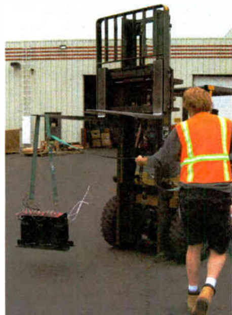
Transformer removed for shipping.
