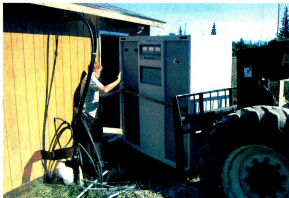
The new transmitter for KBBI(AM), Homer, Alaska, is loaded into the building — with two inches of clearance.
