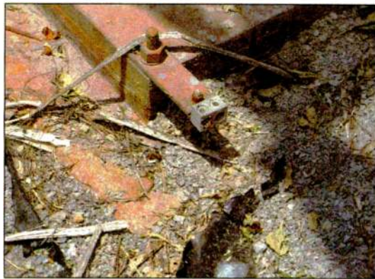
Fig. 1: Missing tower base ground wire makes a site vulnerable to lightning damage.
