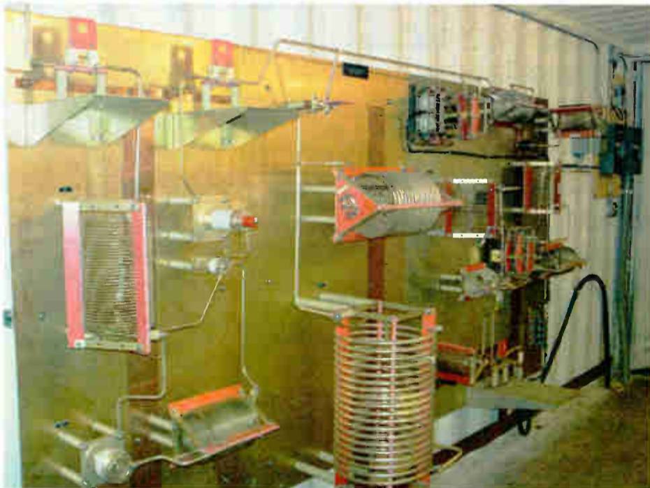
Fig. 1: Make a visual inspection of the site's phasor and ATU.
