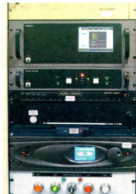
Rack equipment for a typical HD Radio installation, including IBOC generator and audio processor.
