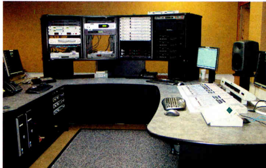
Control Room One in Westwood One's Culver City facility.
