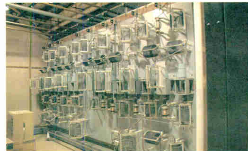
The night phasor network for WISN(AM)'s nine-tower array.
