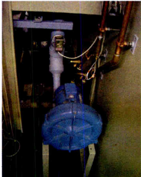
Verify that the air interlock actually works and that air goes to where it is intended to go.
