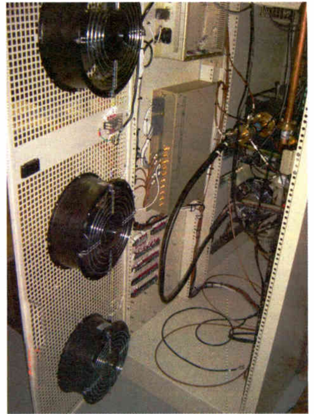
These fans were added to the transmitter door to keep it cool.
