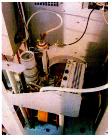
Keep insulators and HV wires clean to prevent arcing.
