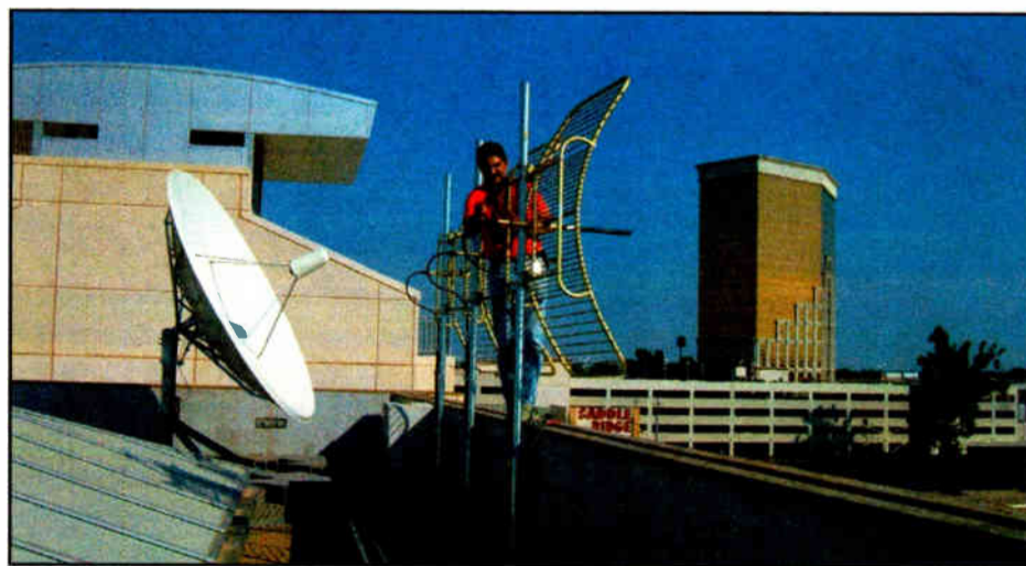
George Walters of Skyline Communications aligns the STL grid antennas.
