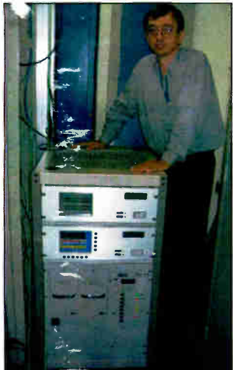
A BE FM-73 transmitter is on the air at KISS(FM) 102.1 in Sao Paulo, Brazil. Engineer Alfredo Marcouizos put the station on the air, the first HD FM signal in Brazil.
