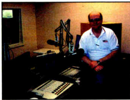
Tom Ray's Axia SmartSurface at WOR is connected to the rack room via a single Cat-6 cable.
