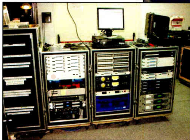
The IBC transmission room featured SAS dual router panels.
