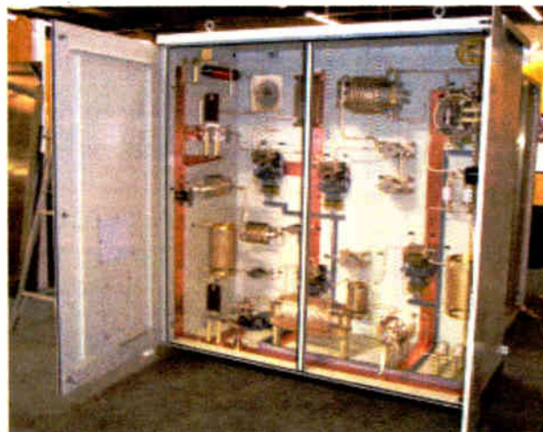
DIRECTIONAL ARRAY ANTENNA TUNING UNIT GAITHERSBURG, MD
