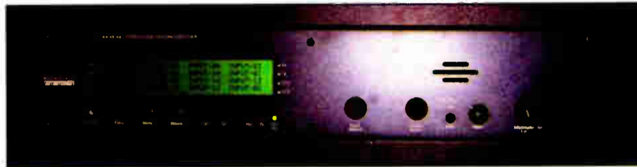
The Broadcast Tools SS16.16 audio router is installed at a Jim Pattison Broadcast Group facility in Alberta, Canada.
