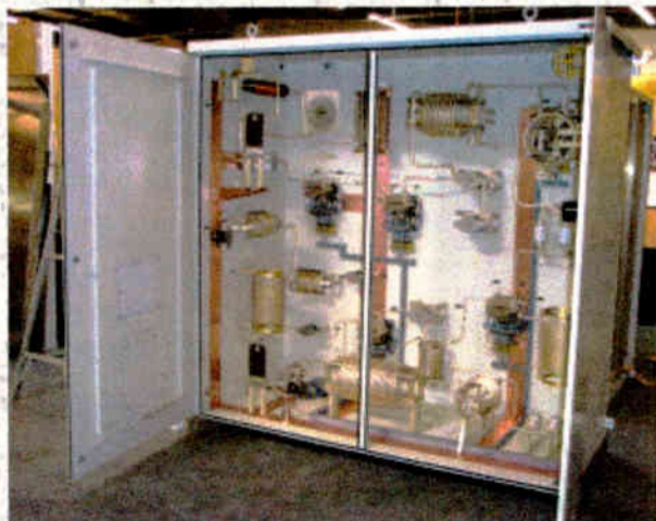
DIRECTIONAL ARRAY ANTENNA TUNING UNIT GAITHERSBURG, MD
