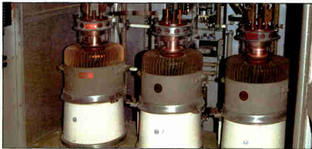
A row of 5671 transmitting tubes in the modulator cabinet of the 50 kW RCA 50F transmitter at WKNR, now WHK, in Cleveland, taken in 2001. The 5671 tube originally was manufactured in large numbers for induction-heating during WWII. After the war they became popular for use in 50 kW AM broadcast transmitters. The earliest version weighed 350 pounds. In later versions, the cooling fins were reduced in number and perforated for more-efficient heat radiation, reducing the weight to 225 pounds.
