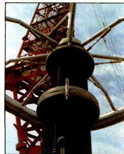
This is a view up through a huge Austin isolation transformer from the foot of the central support tower of the NSS VLF radio station. The transformer is used to couple low-voltage power to the lights on the tower while isolating the RF signal from ground.
