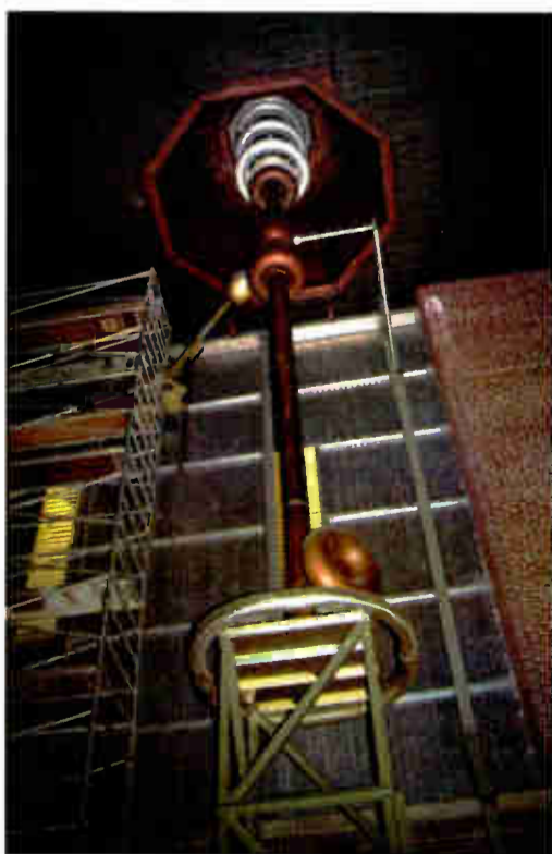
Here's the RF feed in the 'Helix House' at NSS Naval Radio Station in Maryland, shot in 1998. The VLF signal is brought to the top and out of the building to feed a vertical tower at three points. NSS was dismantled in 1999.
