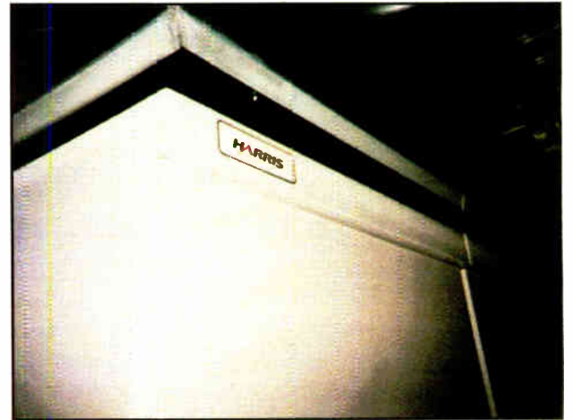
Fig. 2: Ductwork runs to a ceiling exhaust fan. Filtered outside air comes through the rear of the transmitter, heated air exits from the top.
