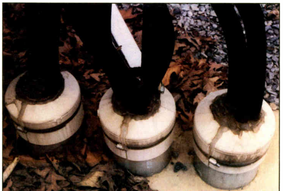
Fig. 3: Here's a slick way to seal PVC conduit that connects a tower to the transmitter building.
