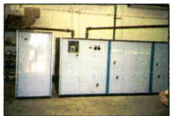
DA Phasing System Cabinet KMJ Radio Fresno, CA 4-Tower 50kW 580KHz
