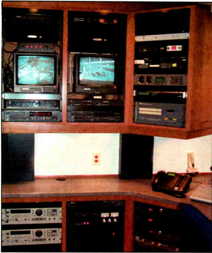
Control Room Left Side
