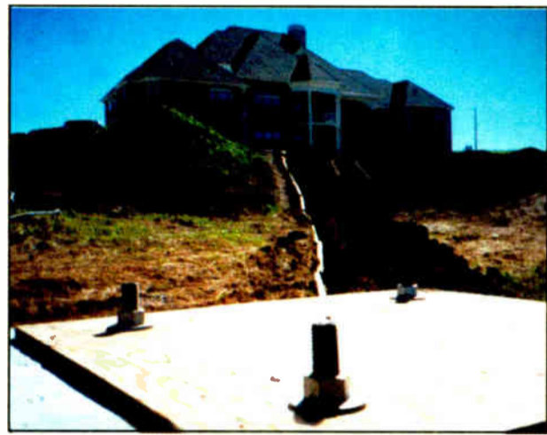
Tower bases and underground feed lines toward the rear of the main building
