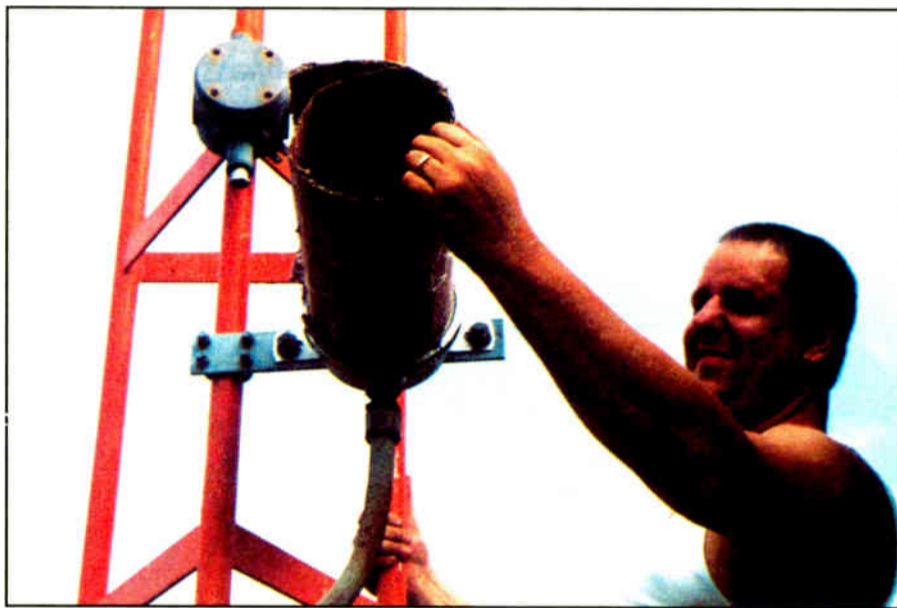
Ray Fantini places the hood over the tower photocell light
