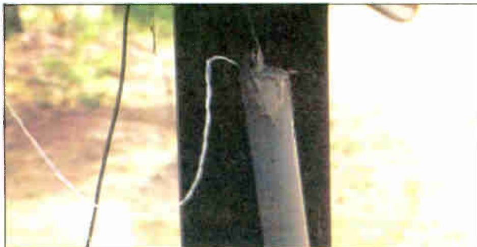
Fig. 2: Sealed conduit with pull string
