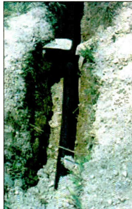
Figure 2: Use caution when trenching in new cable, repairing each cut radial or strap with silver solder.
