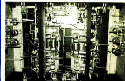
DIRECTIONAL ANTENNA PHASING SYSTEM WMAL-AM RADIO CAP CITIES/ABC WASHINGTON, DC
