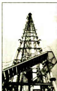
Coaxial Transmission Line
