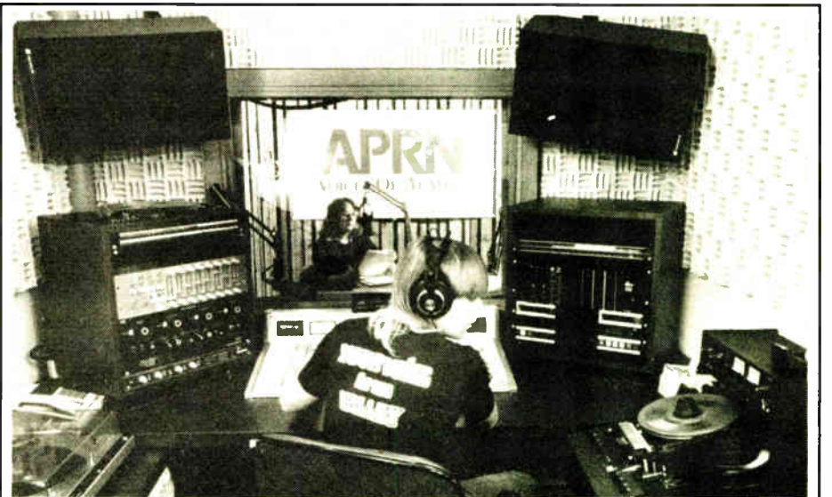
Alaska Public Radio Network built redundancy into its new studio which serves 122 stations.
