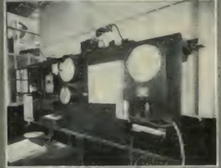
Kiln Control Room
